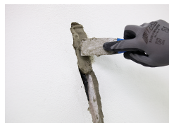
Close the damaged area discreetly.
